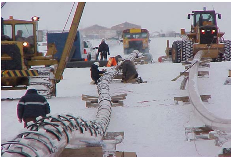
Figure 3.10 – Installing casing insulators on product pipe prior to installation in casing pipe – 4300-foot HDD Colville River Crossing (Source: ASCE Presentation, Michael Baker, Jr. Inc. 1999)
