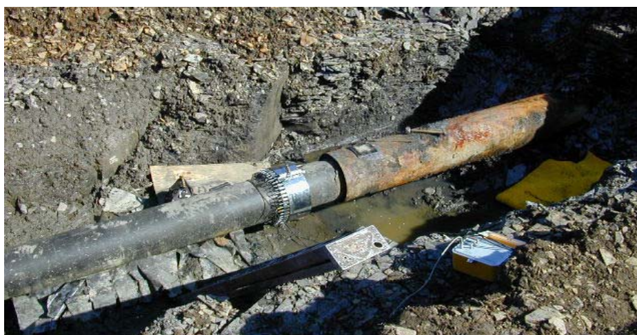
Figure 5.6 – GWUT tool position setup for inspection of a cased crossing (Source: http://www.ultrasonic.de/article/wcndt2004/pdf/guided_waves/818_lebsack.pdf )
