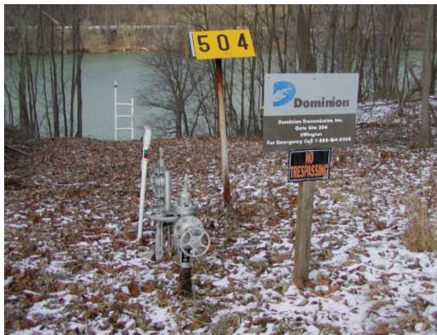
Figure 5.9 – Acoustic system being tested on Dominion line in West Virginia. (Source: http://www.osti.gov/bridge/servlets/purl/838440-wlQSSF/native/838440.PDF )
