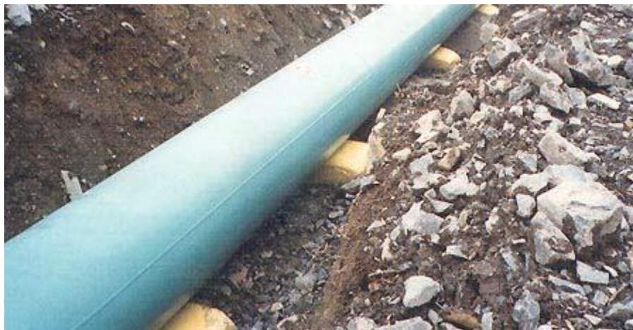
Figure 5.6 – Pipeline on Foam Supports ( http://www.pedero.com )
