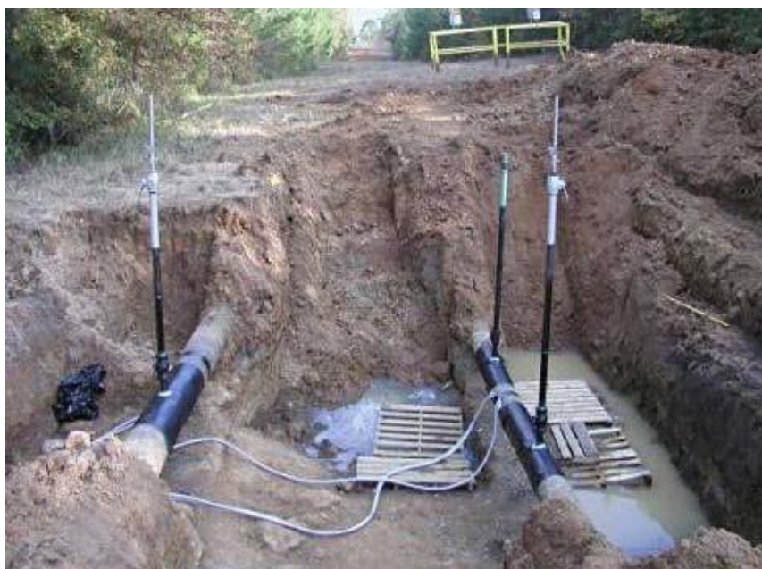
Figure 5.13 – Daylighted Pipeline Site (Courtesy: http://www.process.sensorsmag.com )
